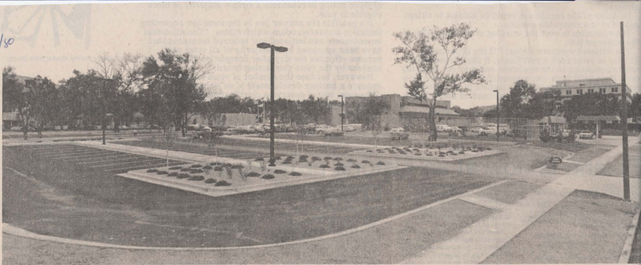
There are 136 parking spaces available in the new lot west of the Public Safety Building (Staff Photo by Don Polovich)
