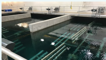
Flocculation Basin at the Jackson Springs Water Treatment Plant. Flocculation is one step in the conventional water treatment process.
